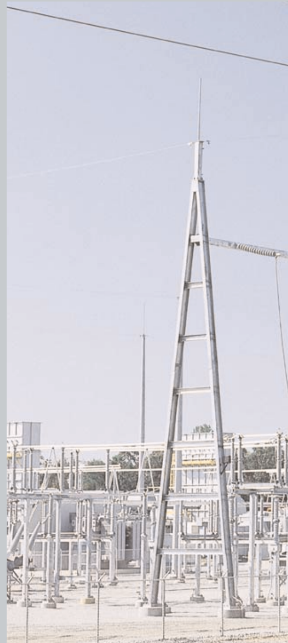
Above, Doyle Substation connects five combustion turbines at a new Monroe, Georgia peaking plant. It consists of two adjacent yards, one with a four-position 230 kV ring bus and one with a five-position 115 kV ring bus.
