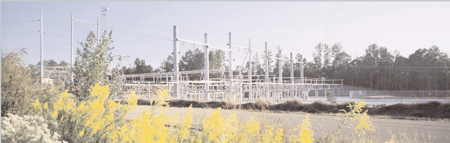
Top, Industrial Boulevard 115-12 kV Substation, Georgia Power Company. Above, Alabama Power’s Crooked Creek 230 kV Switching Station.
